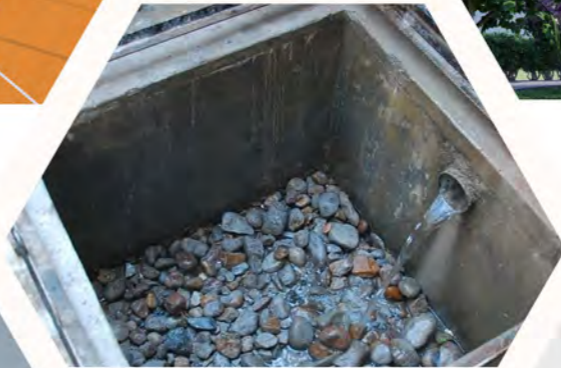
RAIN WATER HARVESTING
